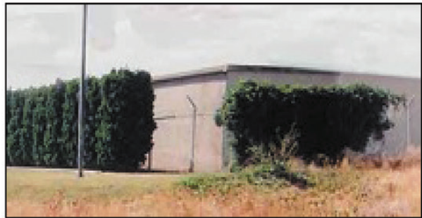
10 Million Gallon Potable Water Tank Pasco, Washington The tank roof eroded from freeze/thaw spalling leaking rain water into tank. Matheson Painting applied Crystal-Lok® to the tank roof solving this problem. Still holding 10 years later.
