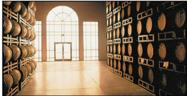
Chateau St. Michelle Winery The Oldest Winery in Washington Required aging tunnels and storage rooms treated for ground water penetration through floors. Done in 1996. No other treatment has been required.
